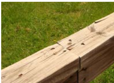
Typical Wooden handrail with exposed nails and splinter hazards
